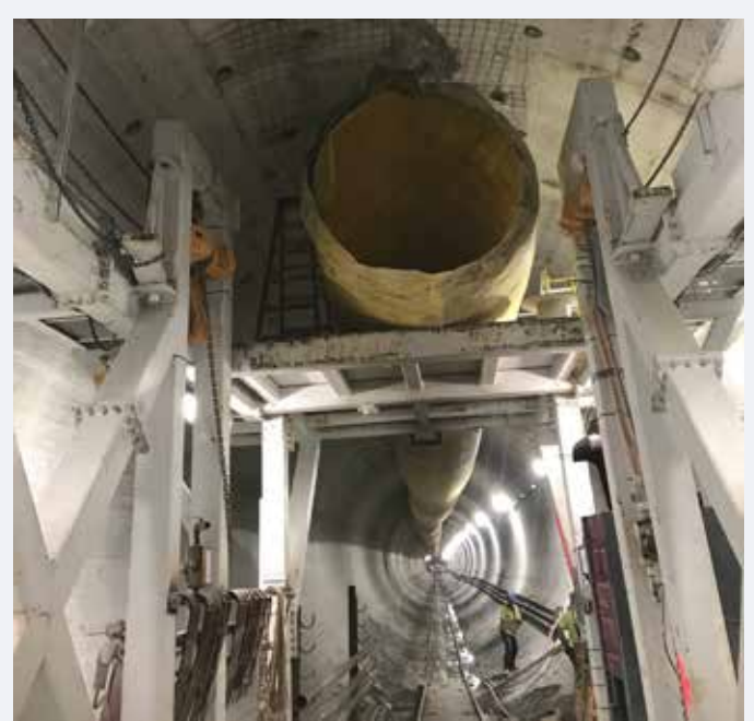
Ventilation shafts pump fresh air to workers who are 200 feet below ground.
