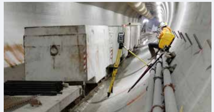
A crew member waits for the muck car train to pass before completing his survey. Muck cars move rock from the boring machine for transport out of the tunnel.
