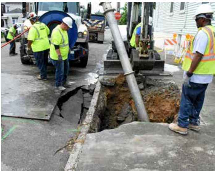
MSD crews work to repair a sanitary sewer cave-in on 25th Street, near the intersection with Main Street.
