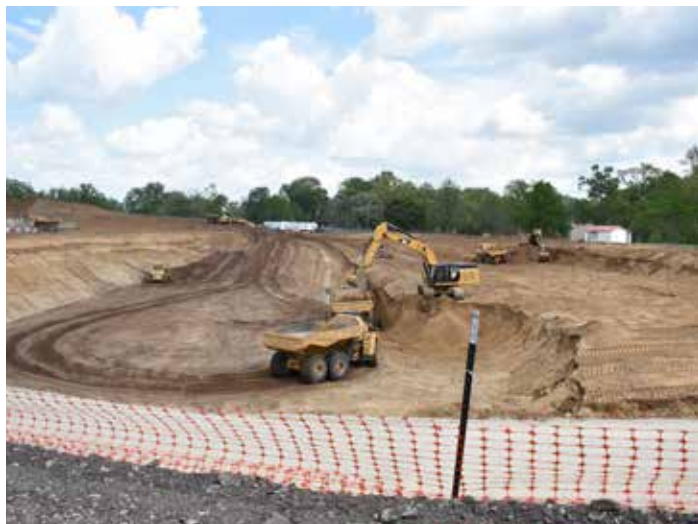
Digging for the Shawnee Park Basin began in early April of this year.
