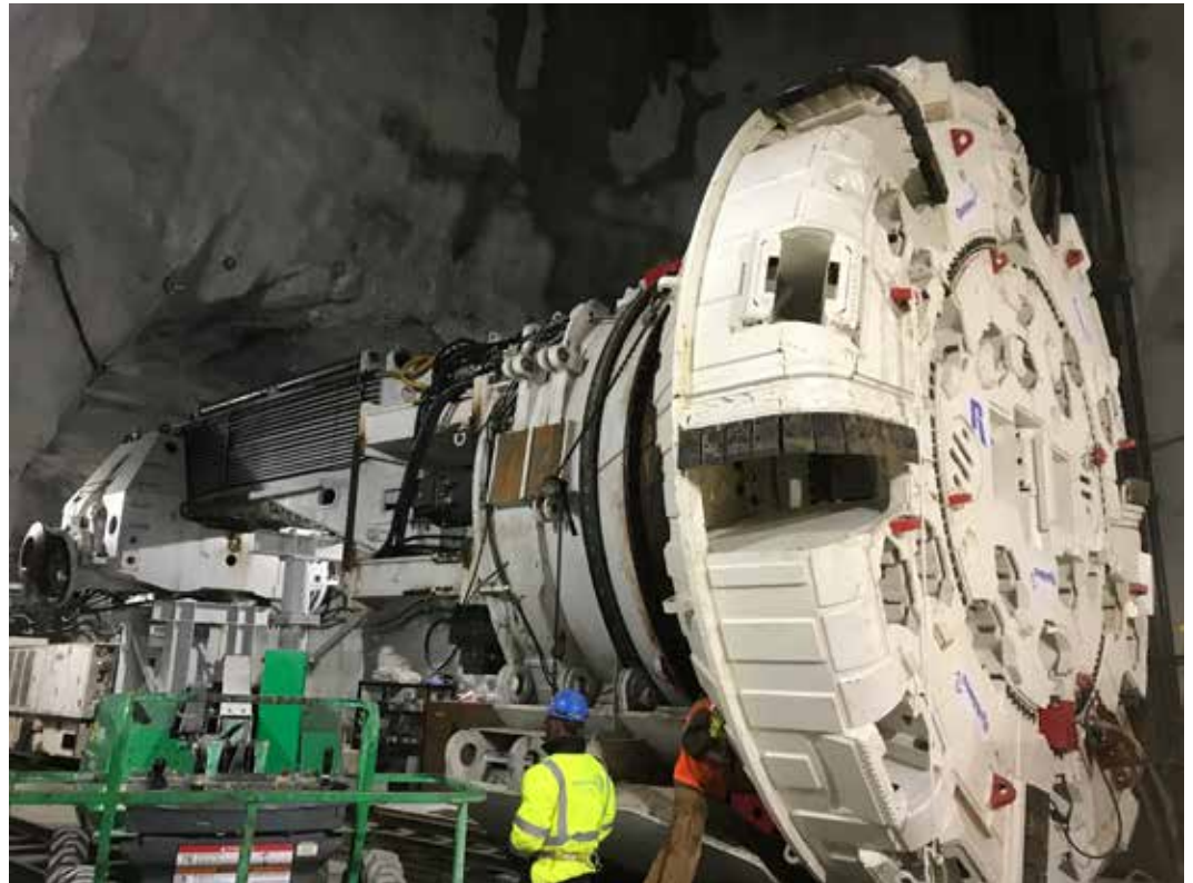
Assembly for Bumblebee’s giant 22-foot diameter cutterhead proceeds underground in preparation for cutting through 4 miles of rock to form MSD’s Waterway Protection Tunnel.
