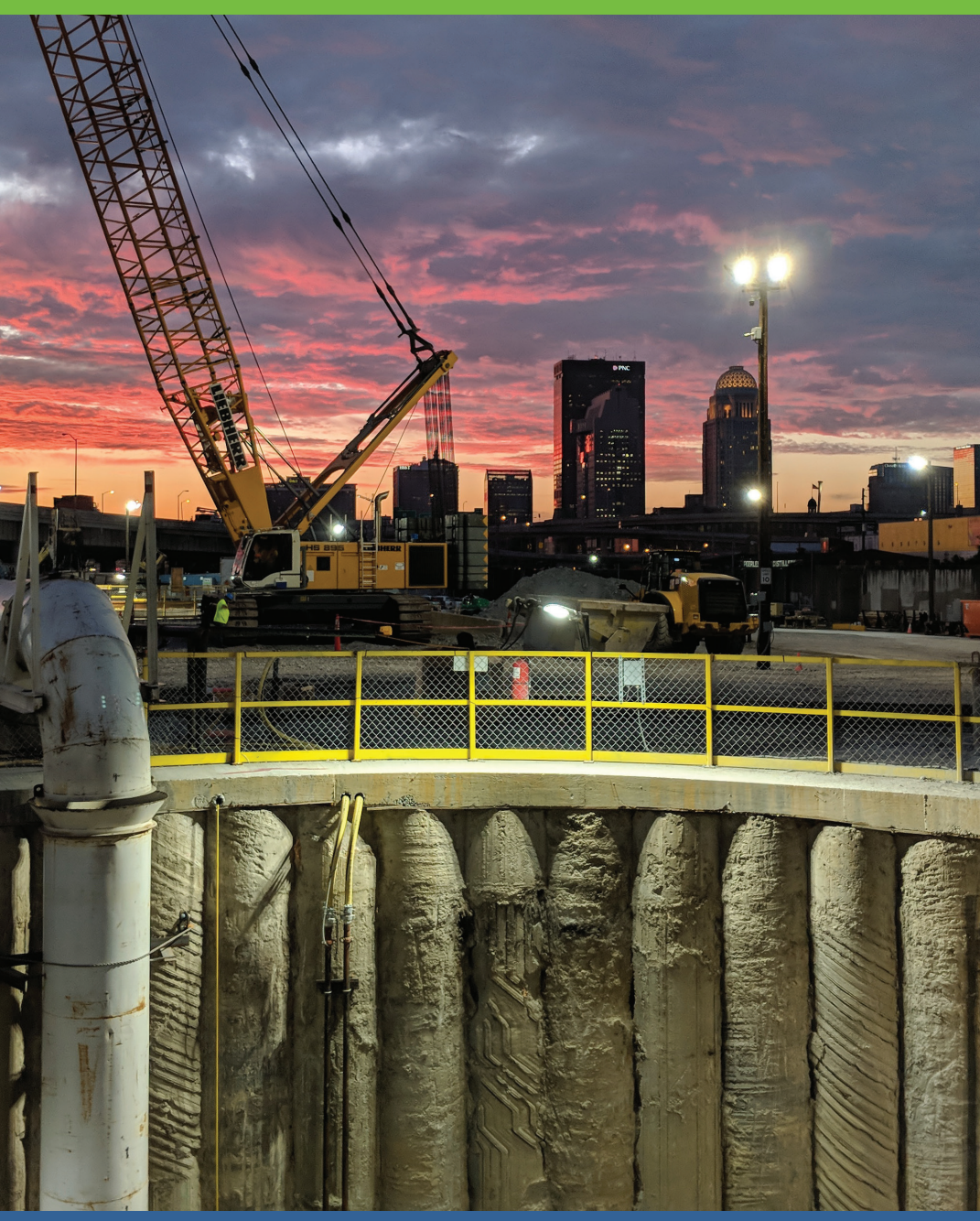
The sky is aglow with morning light at MSD's Waterway Protection Tunnel construction site.
