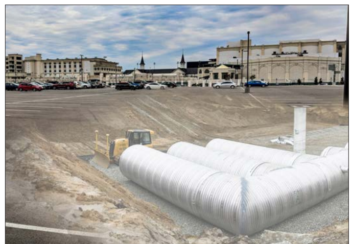
Green Incentive Infiltration Basin at Churchill Downs
