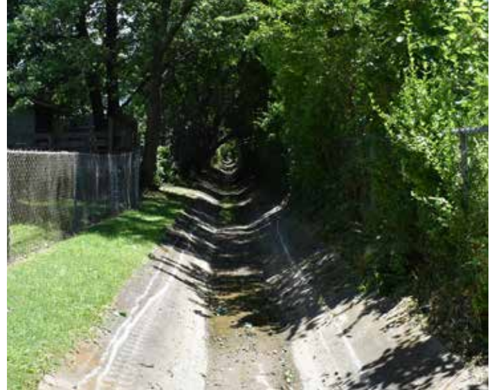
Left, an MSD crew member works to clear plant growth that has obstructed the flow of stormwater. Above, is the newly cleared channel.
