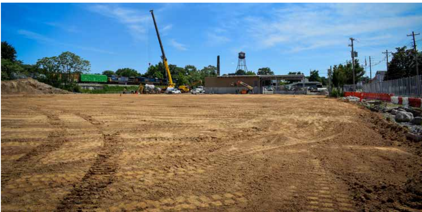
Below: Soil is leveled on the roof of the Logan CSO Basin.
