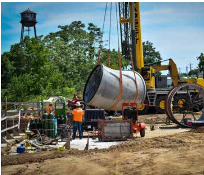
Above: A crane lifts a piece of the Logan CSO Basin interceptor pipe.
