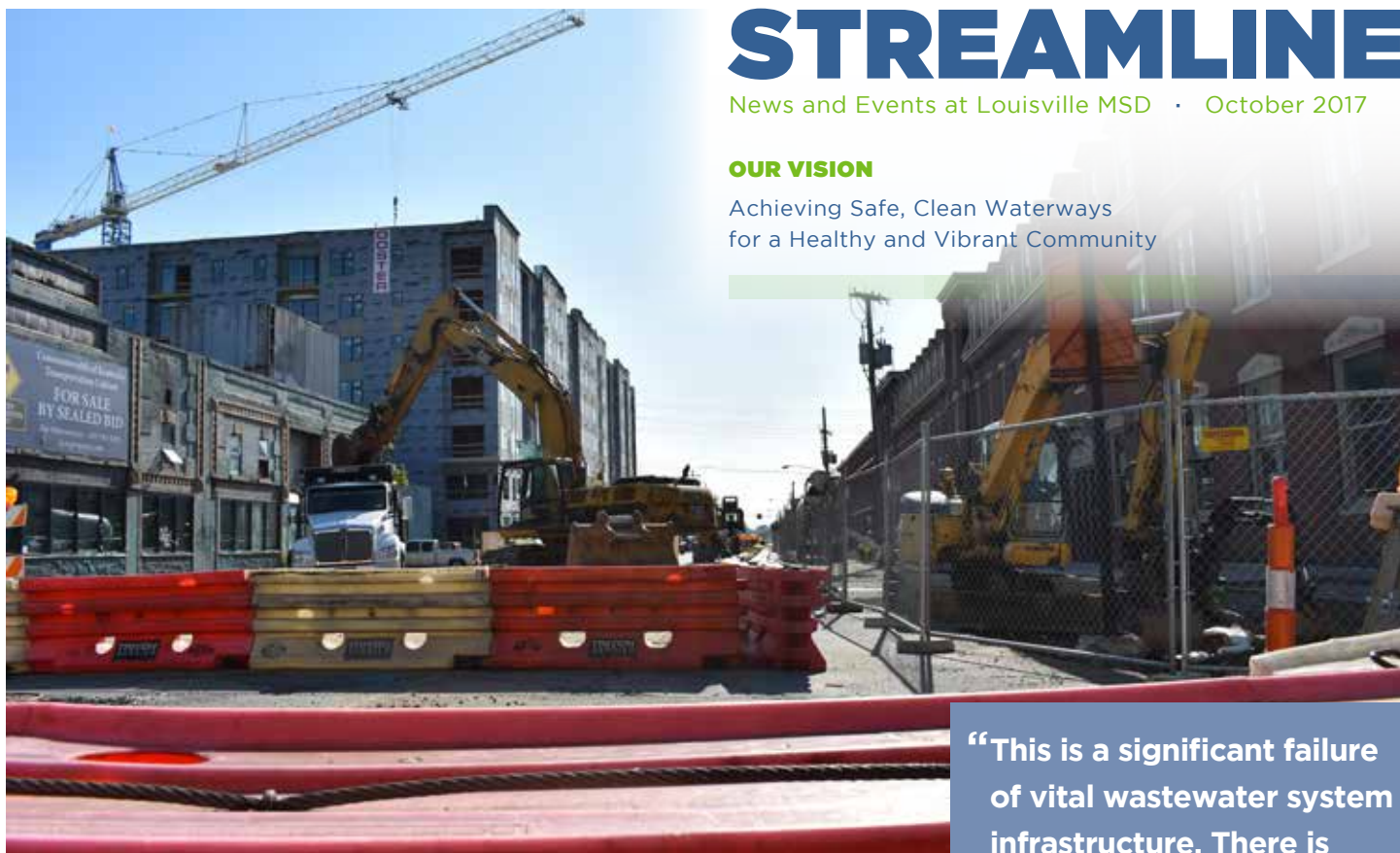
PHOTOS PAGE 1: The intersection of Main and Hancock is the site of a sewer collapse.
