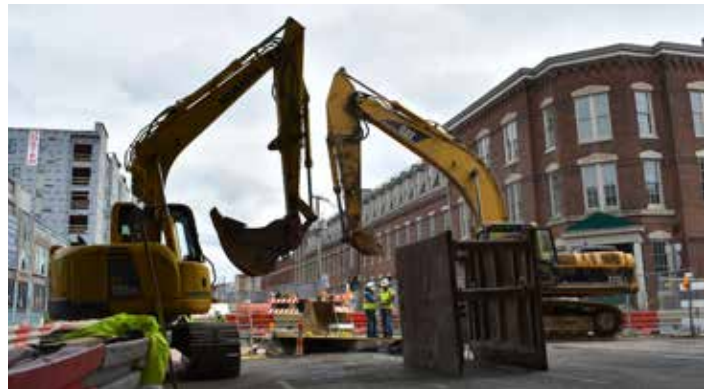
Above: Main Street is full of activity to repair the sewer cave-in.
