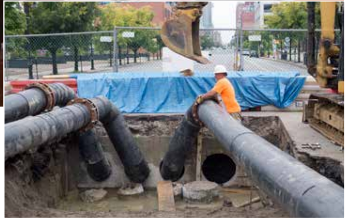
Above: Work continues to complete the connection of the temporary sewerlines into the main sewer system.
