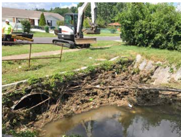
ABOVE: MSD crews begin to clear debris from a drainage channel on Ilex Avenue in the Newburg Neighborhood.
