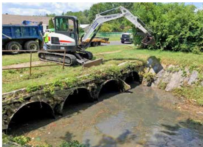
BELOW: The drainage channel was free of debris ahead of heavy rains predicted for September 1 and 2.
