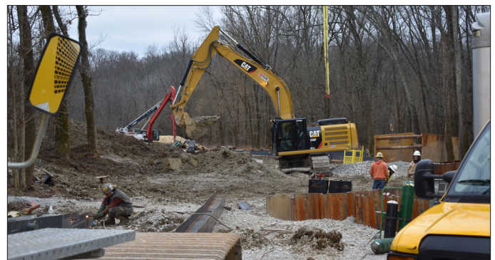
Shaft to access break along Harrods Creek
