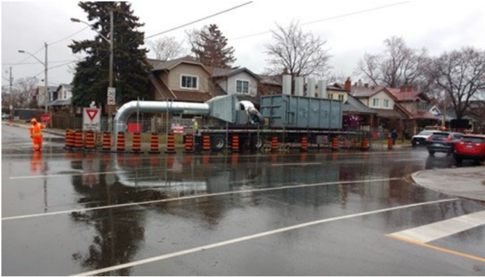
Figure 7 – Example Picture 2 of Negative Pressure Pilot Unit
