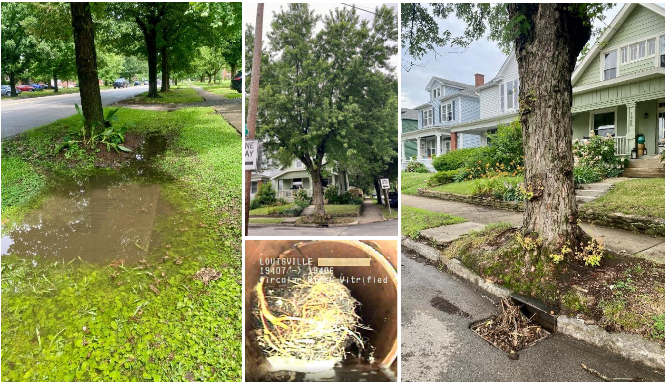
Trees planted too close to drainage infrastructure can cause localized flooding and blockages.
