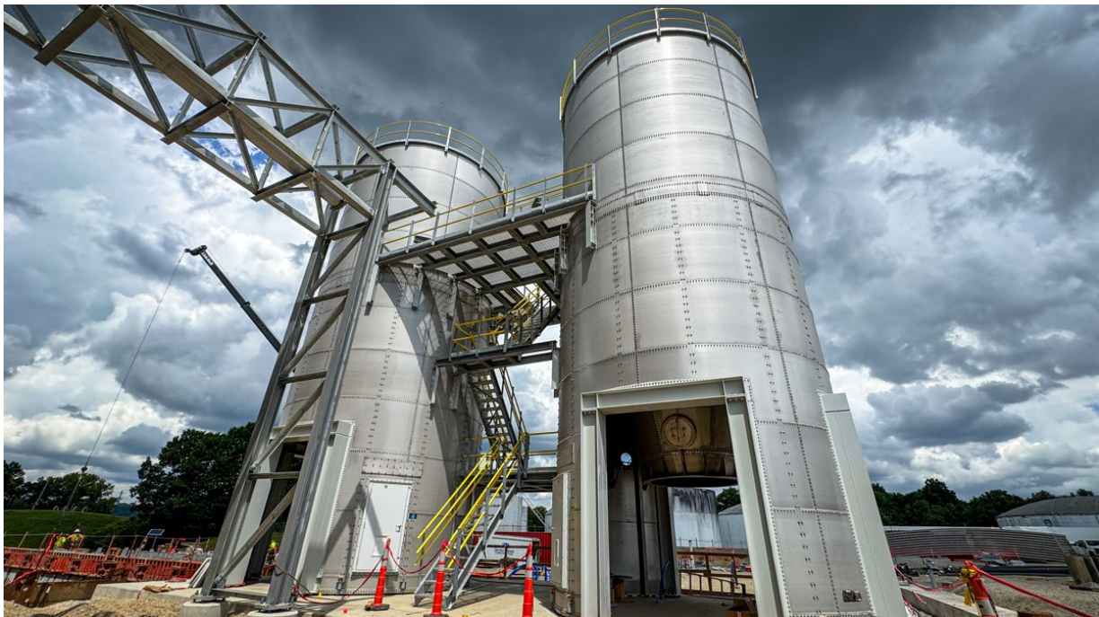
Cake storage silos at the Morris Forman WQTC biosolids facility.
