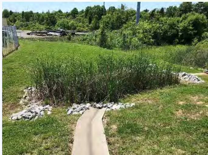
Bioswale at Kentucky Gymnastics Academy
