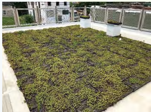
Extensive Green Roof at Healthy House in Louisville, KY
