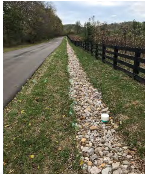
Open infiltration trench in the Parklands at Floyds Fork.
