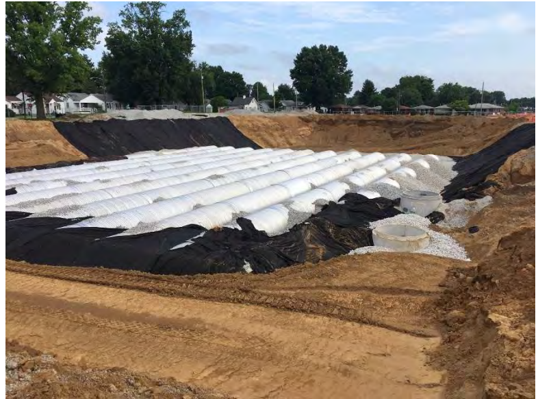
Underground Infiltration Basin at Churchill Downs
