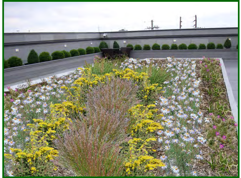
Typical extensive green roof shown during fall blooming season (Concept Rendering: Margaret Shea & Shea Powell, Dropseed Nursery)
