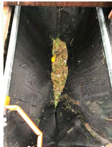
Catch basin insert removes debris underneath an inlet grate on Trade Port Drive.
