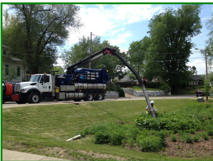
A MSD worker cleans out the inlet structure for a rain garden
