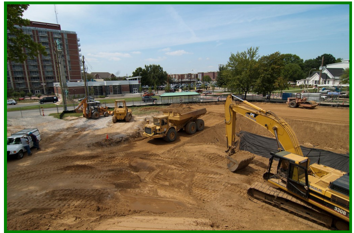
Construction of an infiltration trench at the University of Louisville near the Speed Art Museum
