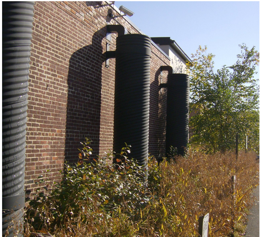
Cisterns drain to a bioswale at the Green Building in Louisville
