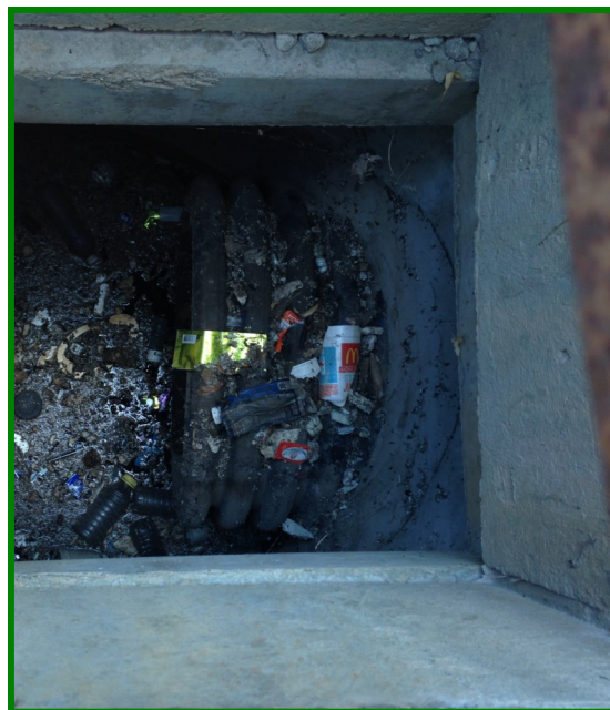
View through the maintenance access port of a proprietary water quality unit shows trash and debris that is separated from stormwater runoff; regular inspection after rain events and maintenance is necessary to clean out these materials
