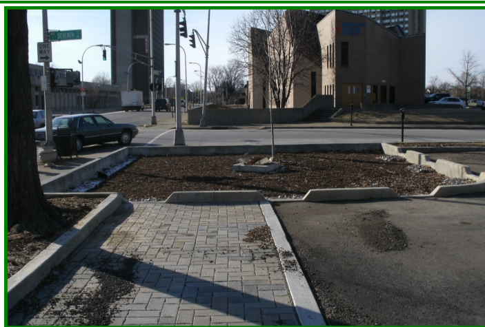
Permeable pavers should be inspected for trash, debris and dirt and cleaned several times per year, as needed
