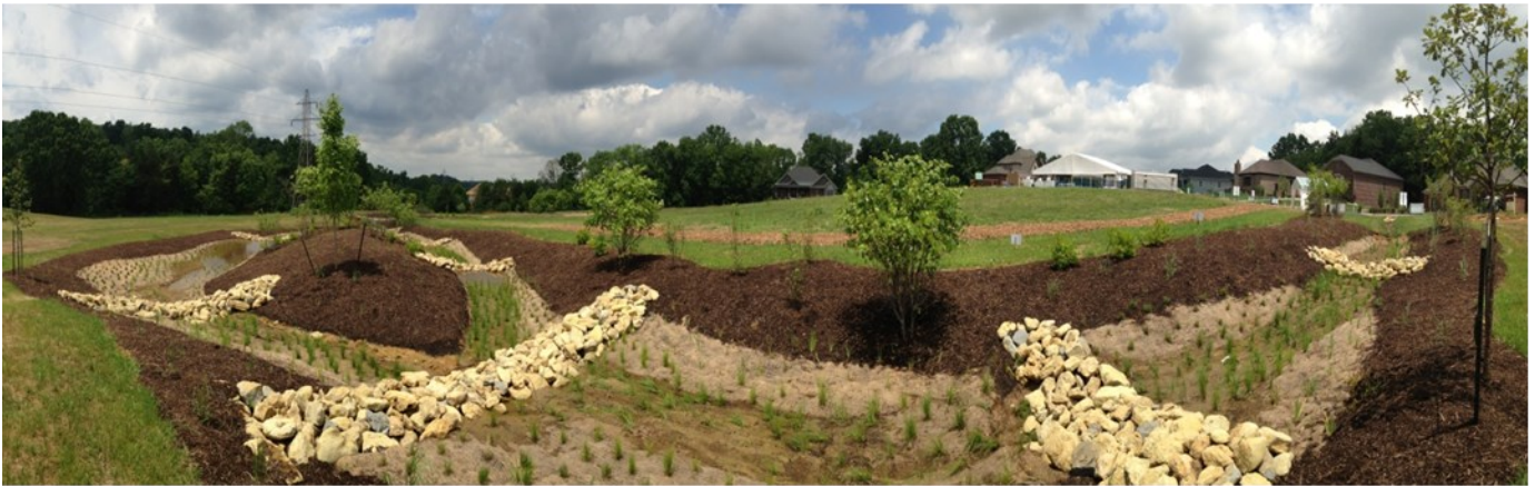
Bioswale with check dams and native plants under construction in a neighborhood development.
