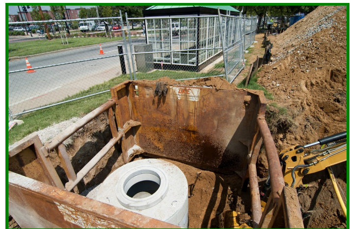
Construction of an infiltration trench at the University of Louisville near the Speed Art Museum
