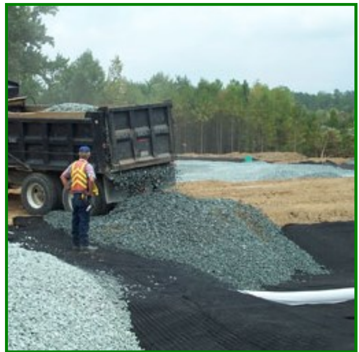
Stone Reservoir with Drainage Pipes
