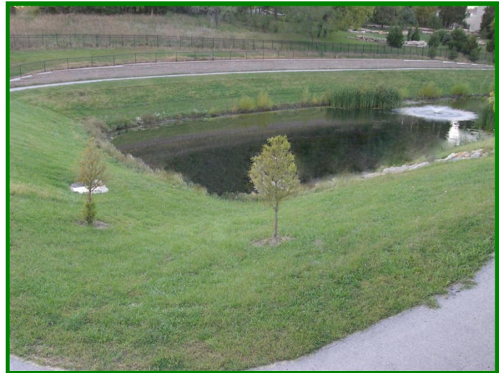
Wet basin with small buffer; trash and debris needs to be removed from the practice to prevent clogging at the inflow and outflow.
