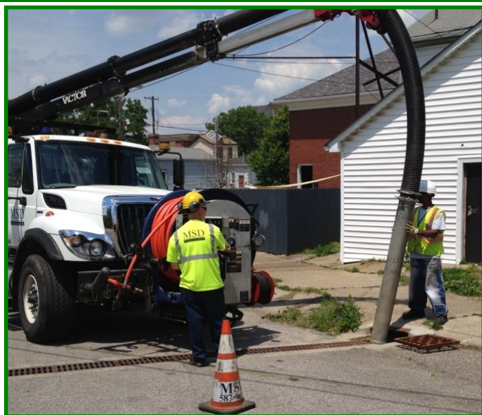
MSD employees use a vacuum truck to cleanout the sump of an infiltration trench
