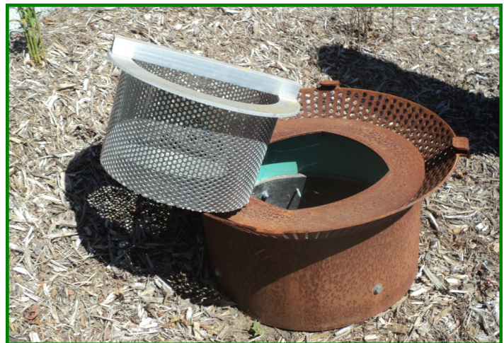
Catch basin inserts should be cleaned regularly to ensure water can flow through the practice and replaced annually
