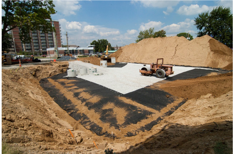
Construction of an infiltration trench at the University of Louisville near the Speed Art Museum
