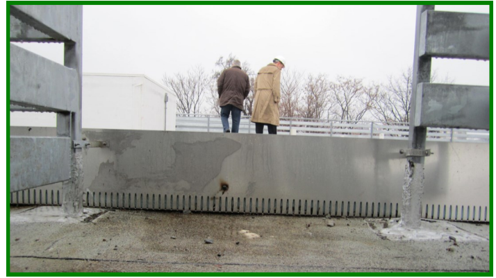
Extensive green roof showing drainage slots and non-vegetated buffer along roof perimeter
