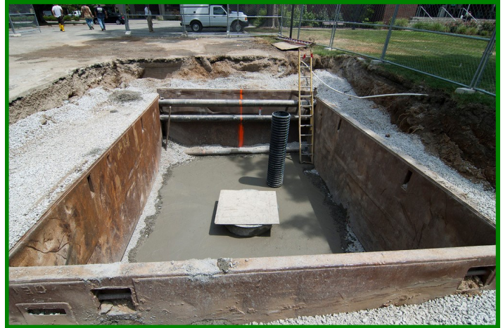
Construction of an infiltration trench at the University of Louisville near the Speed Art Museum
