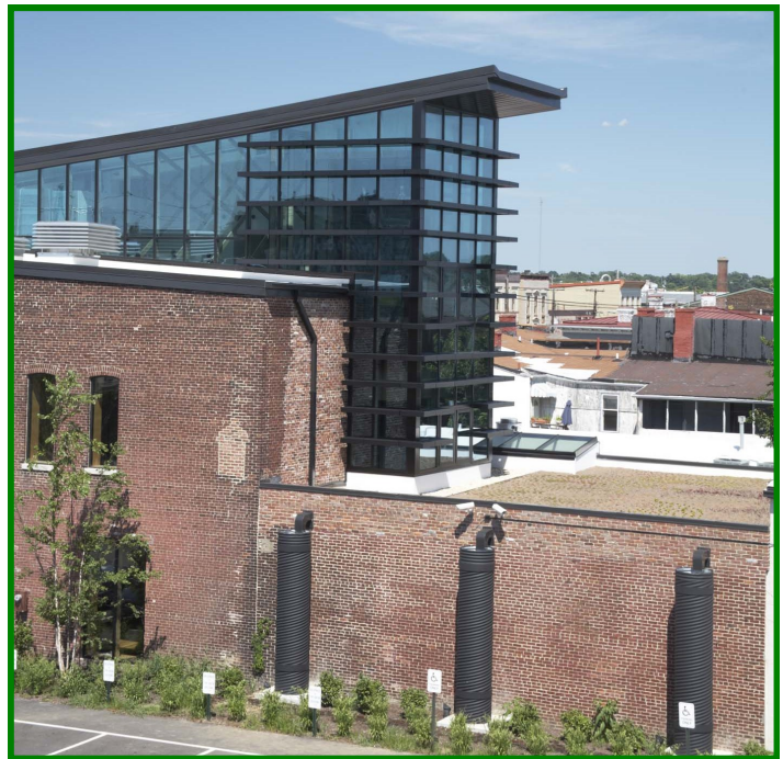
Stormwater treatment train flows from green roof to cisterns to a bioswale
