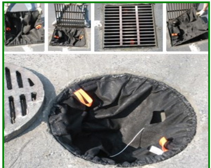
Catch basin insert with an oil-absorbent fabric
