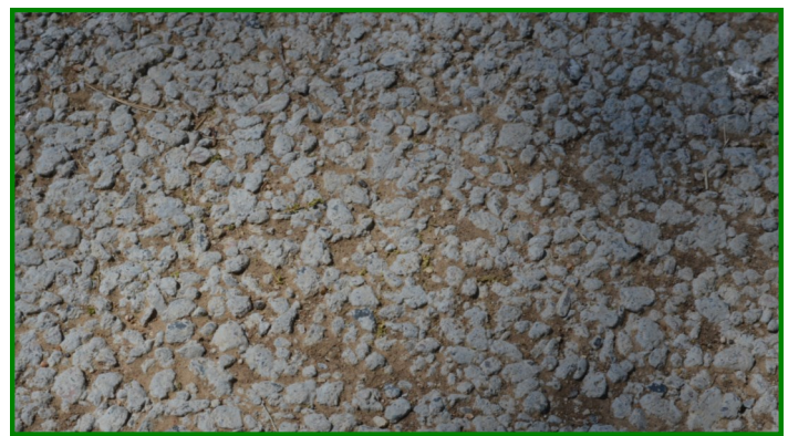
When pervious pavements get clogged, it will be necessary to clean the pavement
