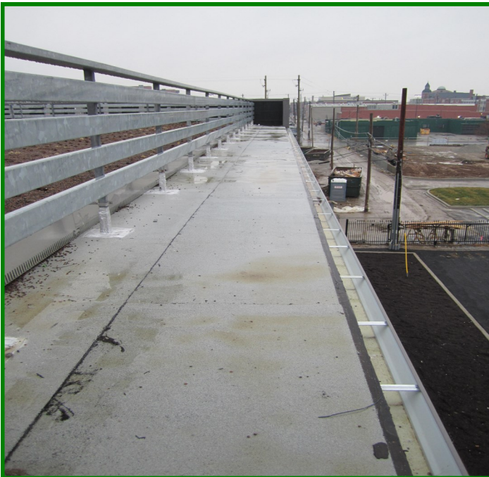
Excess drainage from extensive green roof flows from drainage layer slots over non-vegetated buffer to roof downspouts, which discharge into a rain garden
