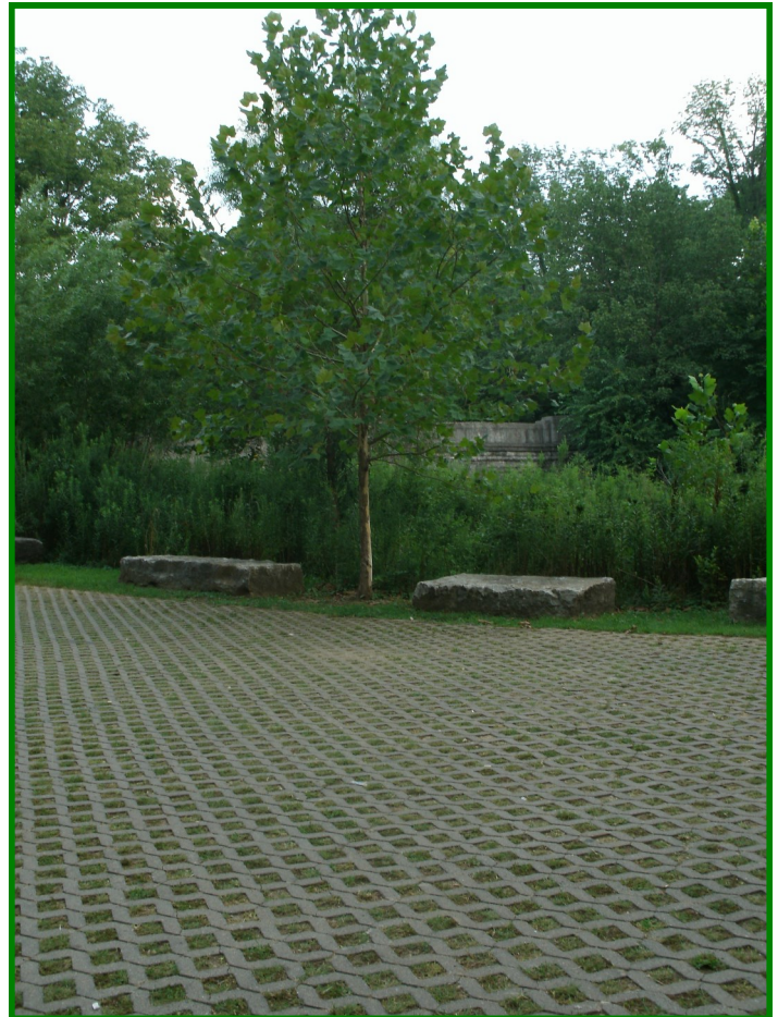
These permeable pavers in a parking lot at Cherokee Park are concrete grid permeable pavers, consisting of a grid filled with topsoil and planted with grass. Concrete grid permeable pavers should be used for light traffic use, such as this overflow parking lot.
