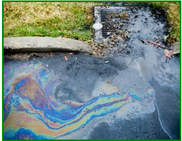
Catch basins should be kept free of sediment, trash and debris and cleaned as needed
