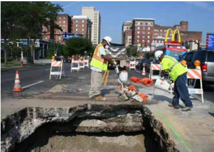
Damien Hughes operates a pavement cutter, while Rontay Winston applies water to cool the blade.
