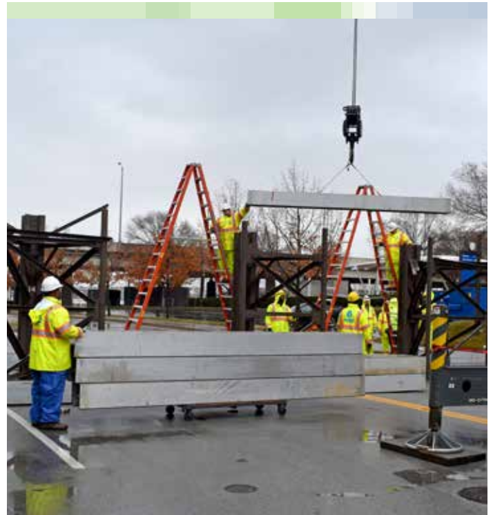
A crane is used to lower pieces of the floodwall roadway closure across Bingham Way.
