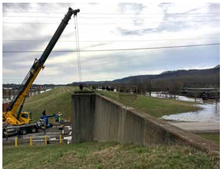
Crews work to install the floodwall roadway closure on Port Road in Riverport.
