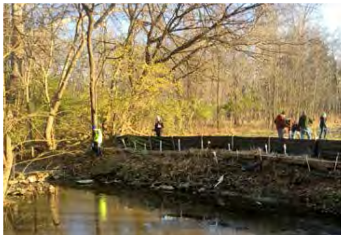
MSD-owned property on Bartley Drive, restored by planting of native trees, shrubs and grasses, will create a forested stream buffer over time that will improve stream health by providing shade and habitat along Cedar Creek. The flood-prone property was purchased through a FEMA grant and the house demolished, per terms of the grant.
