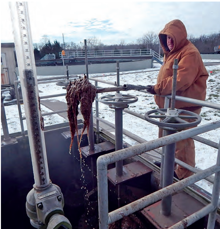
Shawn Smith clears a clog containing flushable wipes at MSD's Cedar Creek Water Quality Treatment Center.
