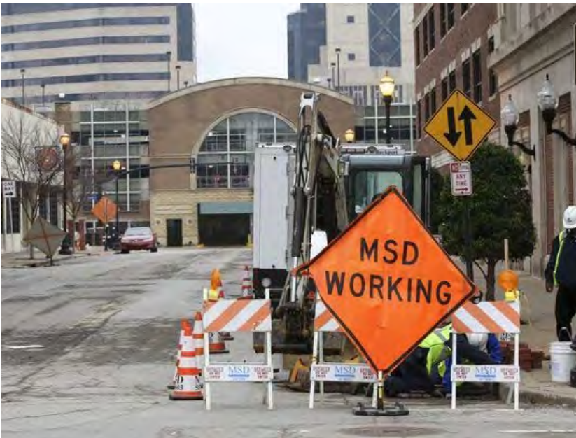
A crew from MSD replaces a catch basin at the corner of 3rd and Guthrie. The basin, made of brick from the late 1800s, has broken down causing a cave in. Jan. 13, 2017 (Photo: Scott Utterback/CJ)
